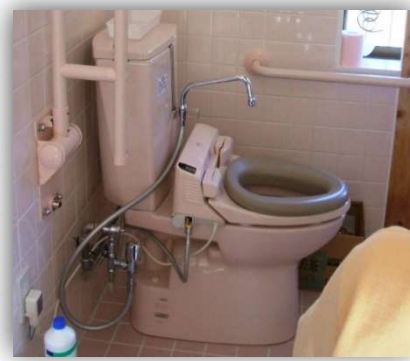
しびん洗浄水栓
