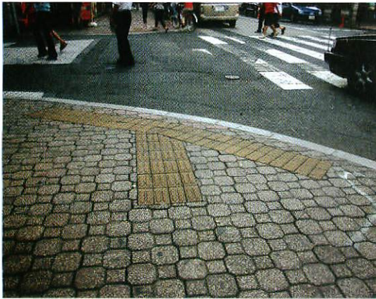
Figure 2-4: Example of road surface with uneven pavers, which makes it difficult for visual impaired people to detect tactile ground indicators
