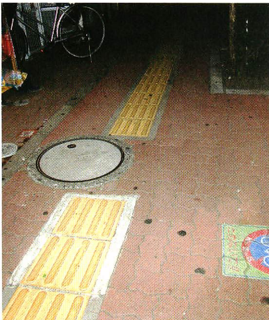
Figure 2-2: Example of stopping tiles on either side of a manhole cover
